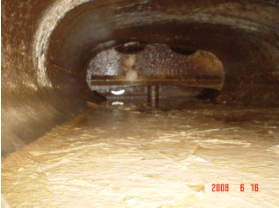
Before treatment with BioTherm Eliminator
